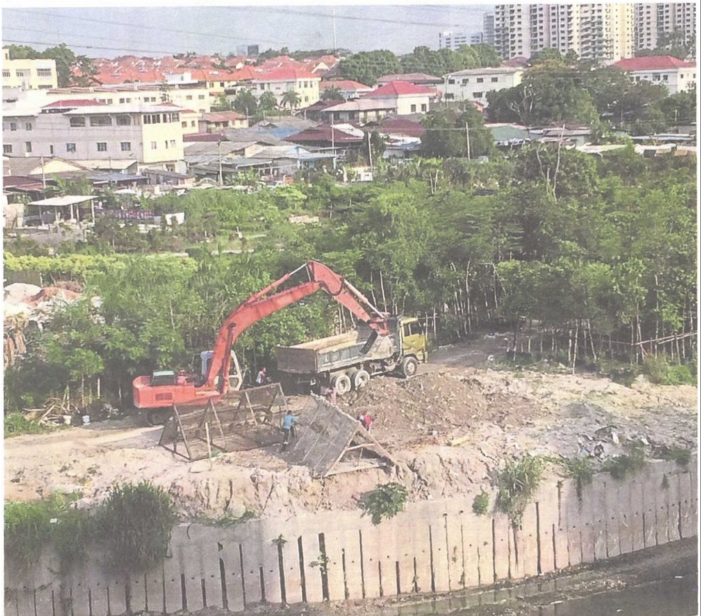
Digging up trouble: An excavator loading sand after it was sifted on the concrete bank, despite a stop-work order by the Selangor Drainage and Irrigation Department to Kumpulan Semesta Sdn Bhd about damaged embankments.
